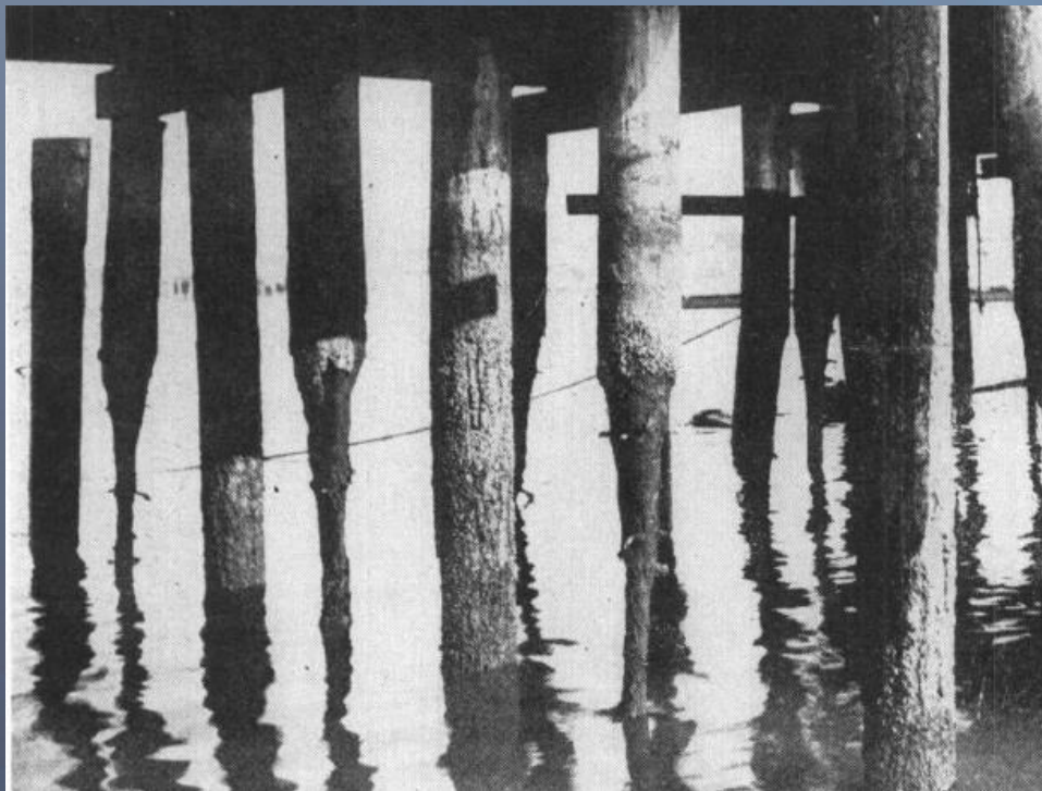
R.J. Menzies, 1957 – Figure 2 ( PDF download ): Pilings destroyed by Limnoria in San Francisco Bay, California. From Hill and Kofoid, 1927 .
